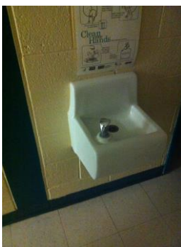
Drinking Fountain needs to be replaced with ADA compliant type
