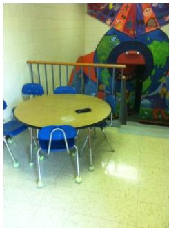
Breakout grouping in fire stair is not permitted
