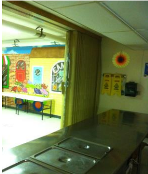
Cafeteria/Kitchen Divider is frayed and should be replaced
