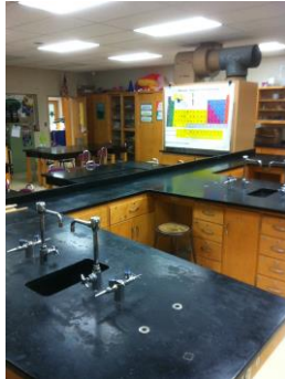
Science casework in poor condition.
