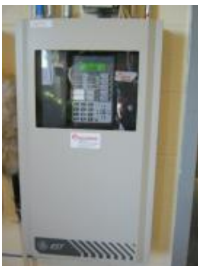
Fire Alarm Control Panel
