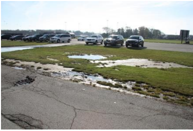
Standing water between drive around school and south parking
