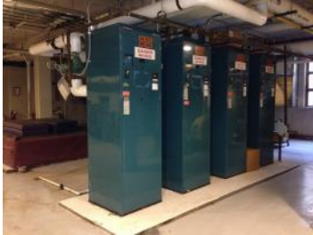
Hot Water Boilers
