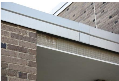
Missing tiles on fascia
