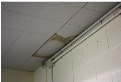
Stained adhered ceiling Tile
