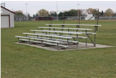
Rusting top rail of bleachers at baseball field
