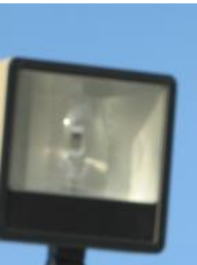
Exterior Parking Lot Pole
