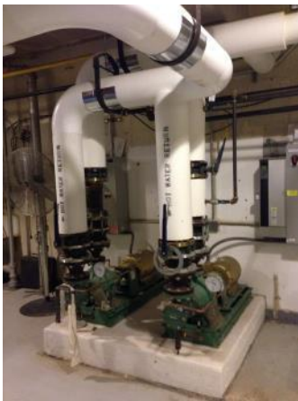
Hot Water Pumps
