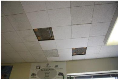
Missing adhered ceiling tile
