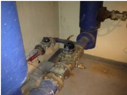
Domestic Water Meter
