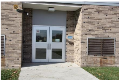
Rusting mechanical louvers
