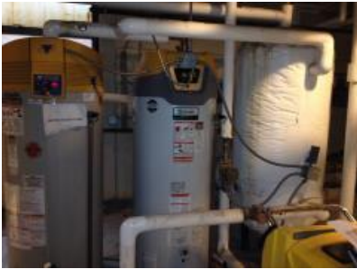
Domestic Hot Water Heating Equipment
