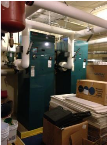
Hot Water Boilers
