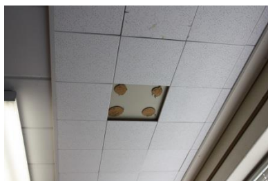
Missing ceiling tile
