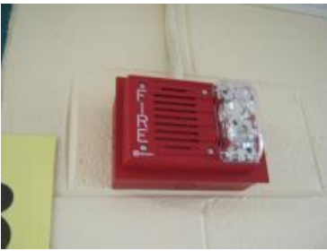
Fire Alarm Notification Appliance
