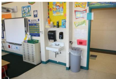
Older VCT in classroom / newer VCT in hallway
