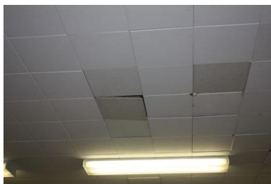
Falling acoustical ceiling tile
