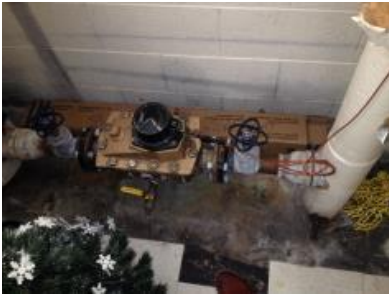
Domestic Water Meter
