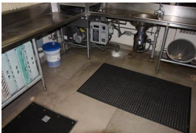
Patched flooring in kitchen
