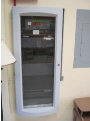
Fire Alarm Control Panel
