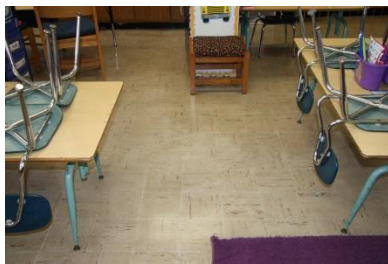
Edges worn on VCT
