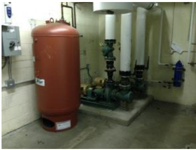
Hot Water System Pumps
