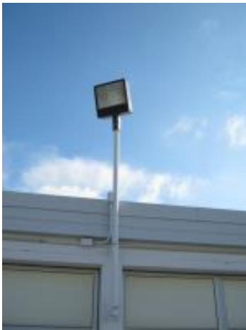
Exterior Parking Lot Pole
