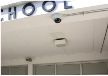
Security Camera system
