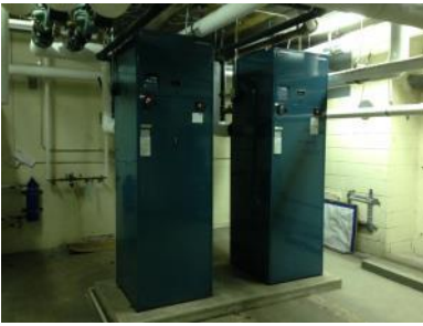
Hot Water Boilers
