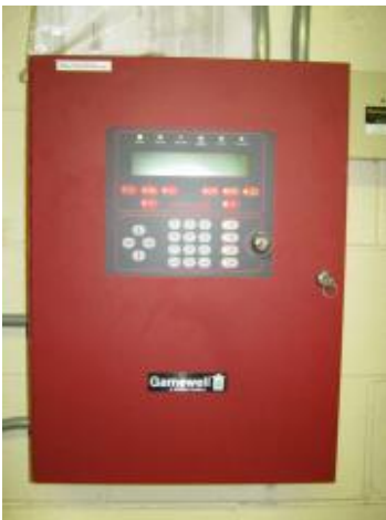
Fire Alarm Control Panel
