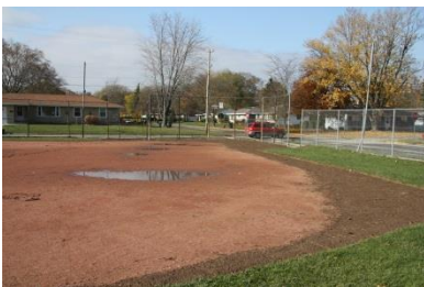
Ponding water at baseball field
