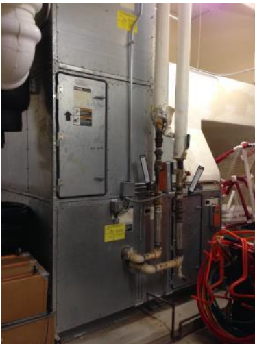
Hot Water Air Handling Unit
