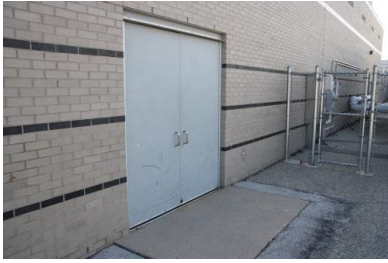
Dented and rusted steel door
