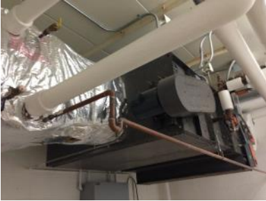
Lower Level Air Handling Unit
