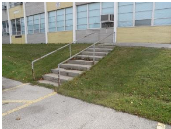
Rusted metal railing
