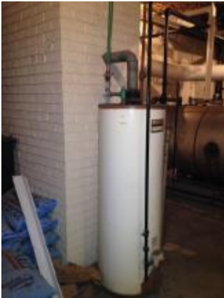
Gas-Fired Water Heater
