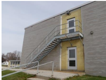
Rusted metal stair
