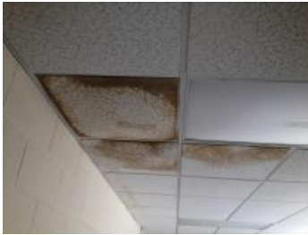
Ceiling tiles indicating water leaks
