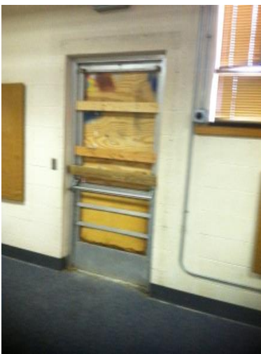
Boarded up aluminum door
