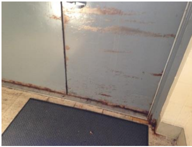
Dented and rusted steel door
