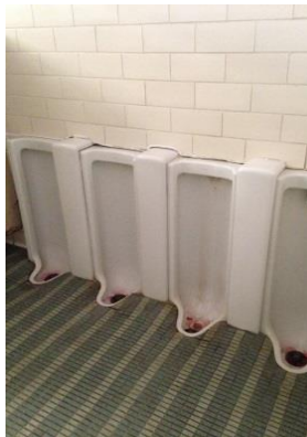
Urinals in boy's restroom
