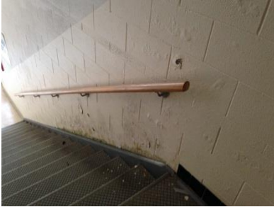
Southeast stairwell water damage
