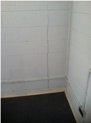
Crack in concrete blocks
