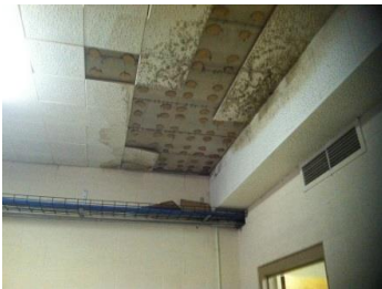
Missing ceiling tiles and Mold
