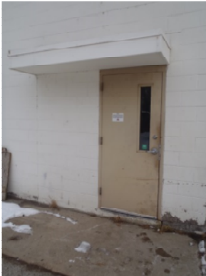
Rusted hollow metal door frame
